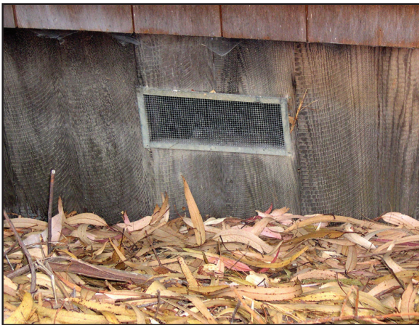
Combustible material like this mulch, near skirting or siding, leaves the home unprotected, even with screening in place. Photo by Institute for Business and Safety Research Center.
