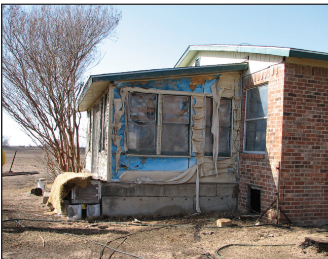
The vinyl siding and window frame on this home melted when exposed to radiant heat.
