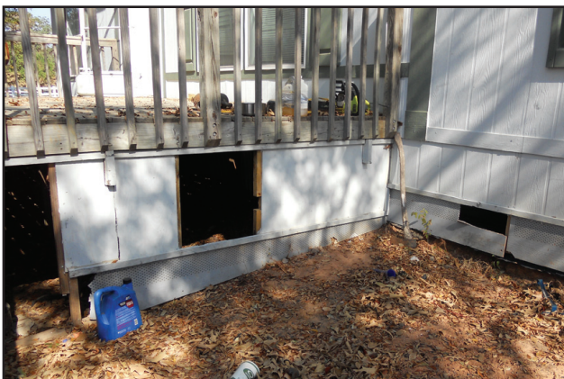
The flammable skirting under this deck, along with mulch, could easily lead flames to the deck and home.
