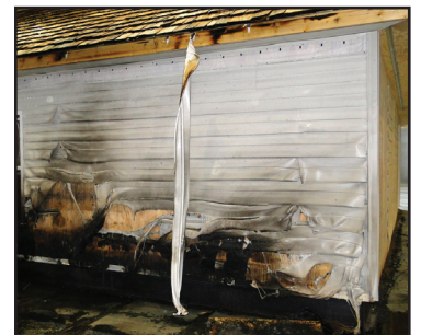
This vinyl gutter melted from heat, exposing the wood and roof edge to embers and direct flame. Photo by Institute for Business and Safety Research Center.
