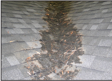
The pine needles on this roof burned, but the Class A roof did not. Photo by Institute for Business and Safety Research Center.
