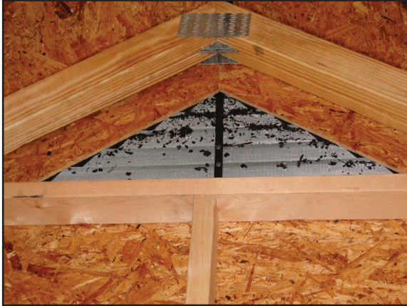
Screening helped capture these embers and prevent their entry into the attic. Photo by Institute for Business and Safety Research Center.
