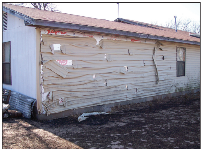
When this vinyl siding melted, it exposed other combustible materials.
