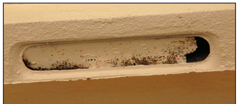
Vents can clog. This vent was painted over, reducing its effectiveness in providing ventilation. Photo by Institute for Business and Safety Research Center.
