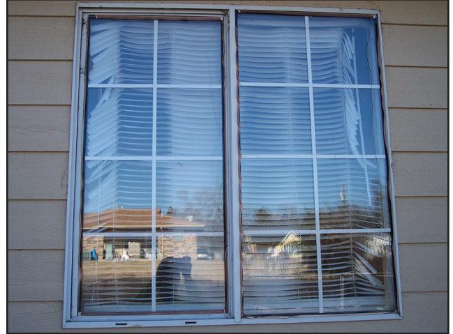
Radiant heat melted the interior blinds.
